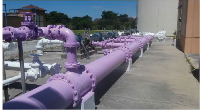
Purple pipe is used to designate reclaimed water and separate it from potable water. (Image Source: Brown and Caldwell)
