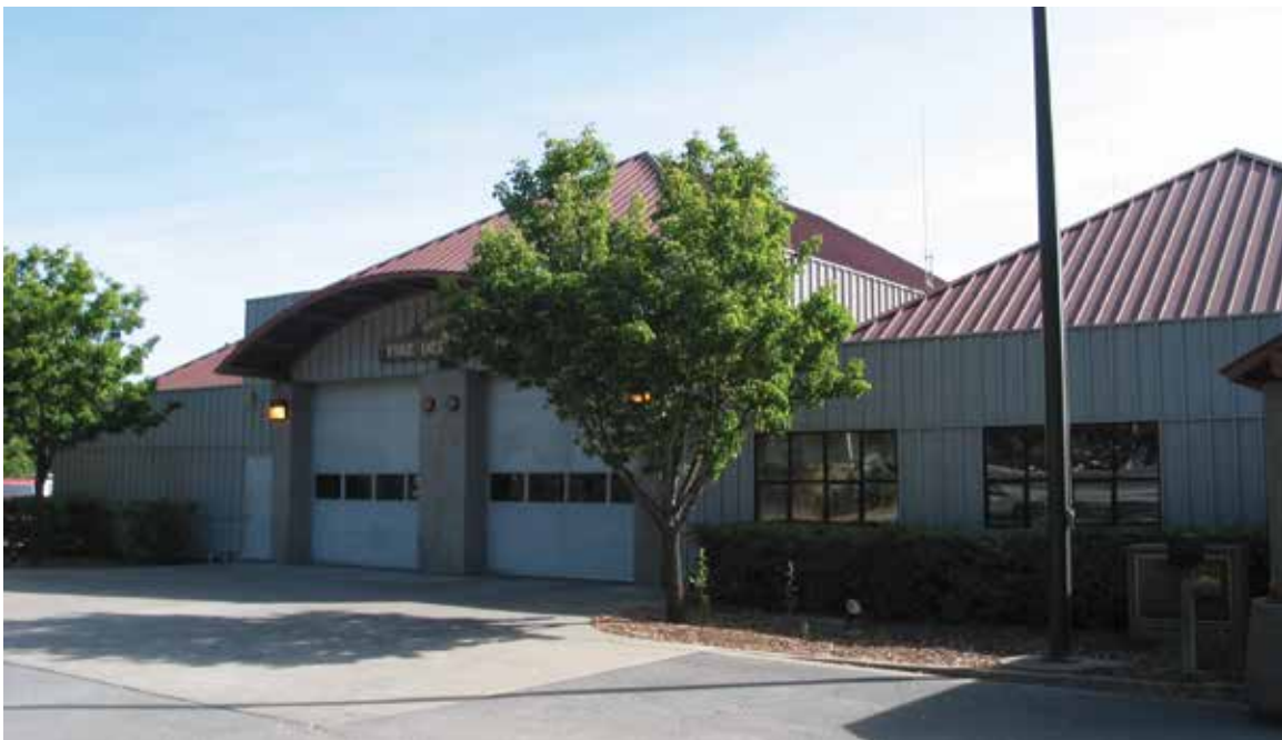
Brisbane's new fire station, on Bayshore Boulevard, was dedicated on May 9, 1992. Unfortunately, roof leaks eventually led to mold problems that forced firefighters into temporary quarters next door until repairs were made.
