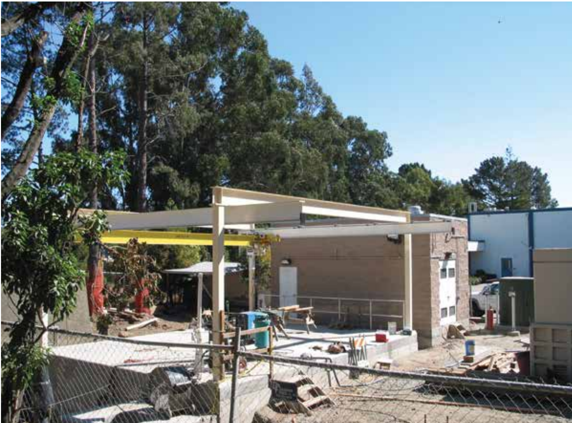
City Manager Clay Holstine and City Engineer Randy Breault had long recognized the danger to Brisbane of flooding posed by an outdated pumping or "lift" station on Valley Drive, near City Hall and the Community Park. They oversaw a major upgrade in 2003, and in December of that year the Valley Drive Lift Station proved its worth, handling 3.1 million gallons per day of runoff during a heavy storm.
