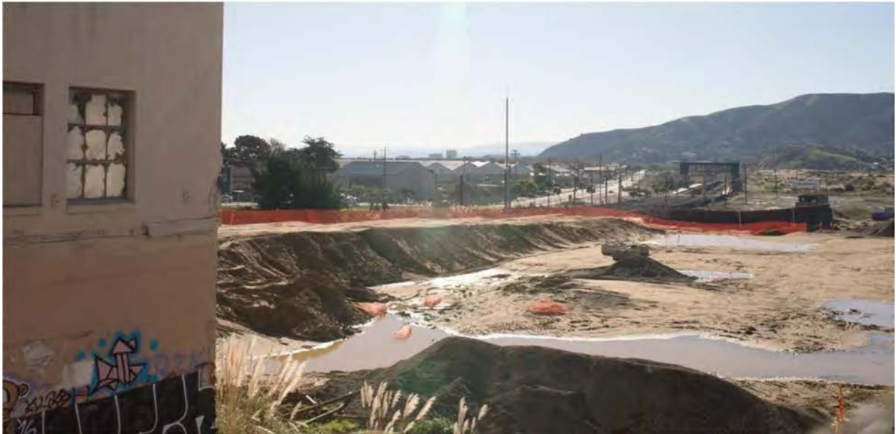
Draft EIR/EIS Figure 3.15-22: View of Bayshore Caltrain station from the Schlage Lock construction site.
