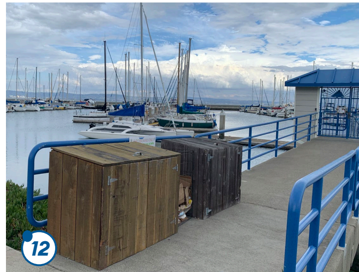
12 Access to docks is via concrete gangway with a locked gate. Trashcans at the head of each gangway are publicly accessible and suffer from vandalism and possible animal interference.
