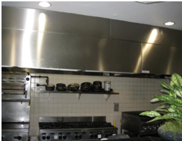
Figure 37 – Kitchen exhaust hoods
