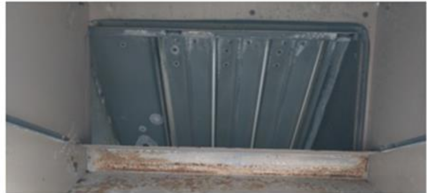
Figure 31 – Example of a mechanically fixed outside air damper
