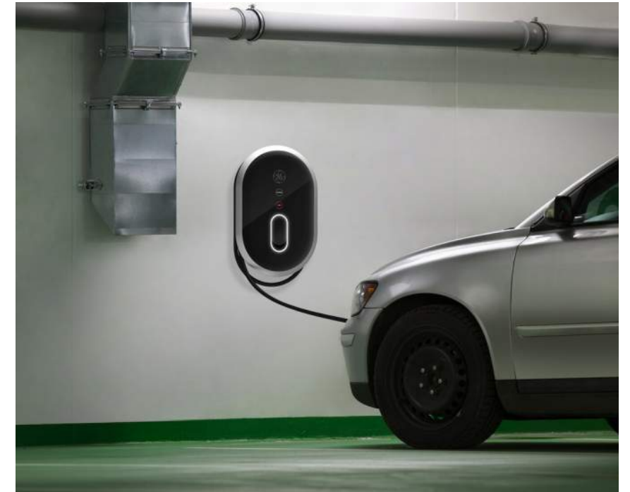
Electric car charging stations shall be installed per CALGreen requirements.
