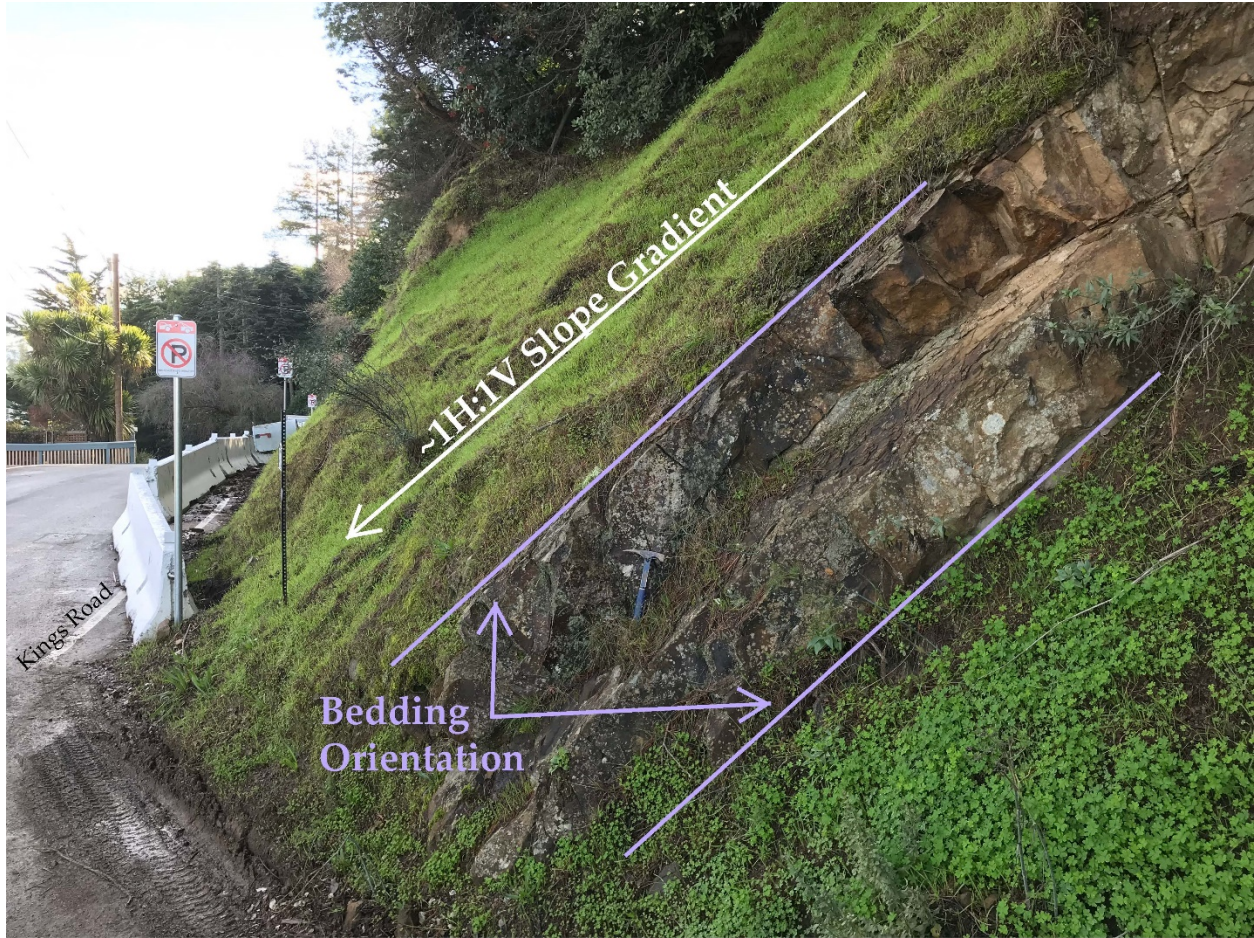
Figure 3: Photograph taken from Beatrice Road facing southeast towards Kings Road. In the fore-ground, fractured sandstone and shale bedrock of the Franciscan Complex is exposed on the slope. It appears that a previous rock-slope failure along a bedding plane (orientation annotated in purple) may have exposed this bedrock outcrop. Colluvial slopes are inclined at grades of approximately 100 percent (1H:1V Slope Gradient).
